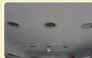
Rear A/C Unit with 6 Roof Vents
